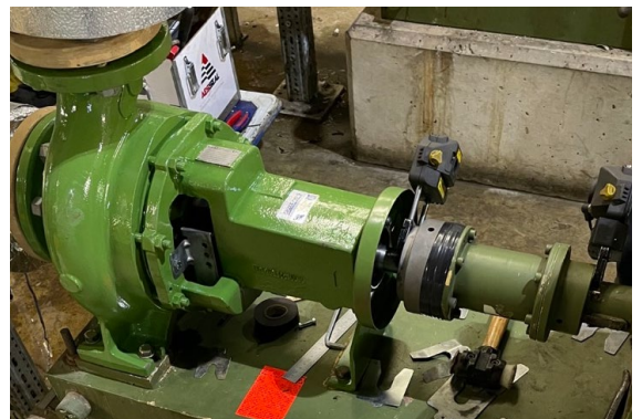
KSB ETANORM PUMP AFTER
